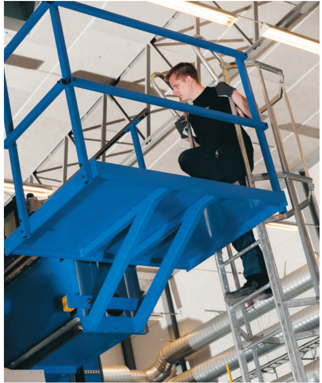
Access to the top of the gantry through service ladders with a platform.
